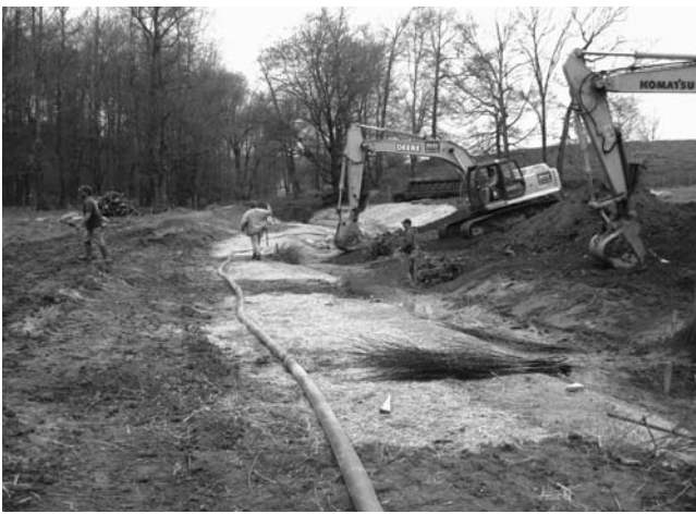
Engineers work to recreate a meandering stream by laying out the stream bed and re-sloping the banks.
