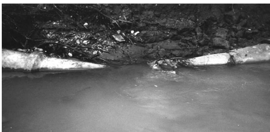
Infrastructure failures, such as the broken pipe above, are more costly to repair than they are to prevent.
