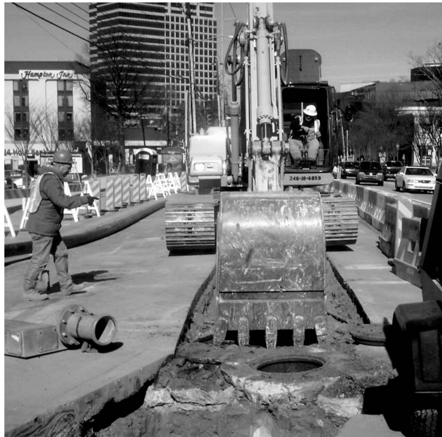
City workers use pipe-bursting, a trenchless method of pipe reconstruction, on Piedmont Road in Atlanta.
