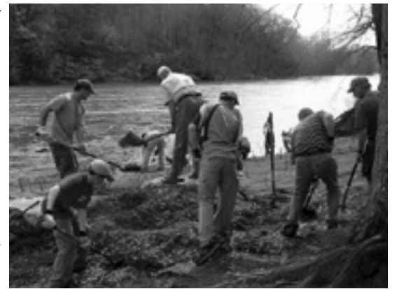
Volunteers work hard to stabilize the eroding bank next to the main stem of the River.
