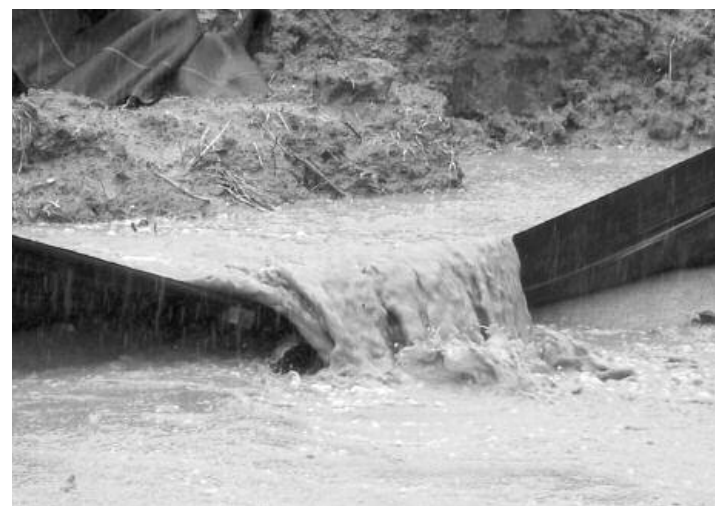
This overflowing silt fence was poorly designed or not maintained, allowing muddy water to flow into nearby streams.
