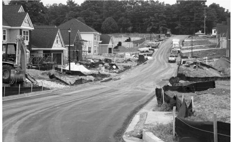
Sediment enters the street and storm drains in this Douglas County subdivision where best management practices do not meet state regulations.
