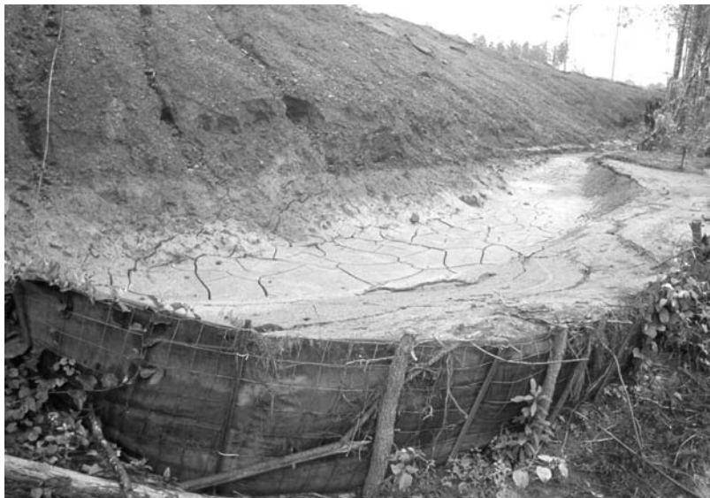
Silt fence full of mud at a subdivision site constitutes an erosion violation.
